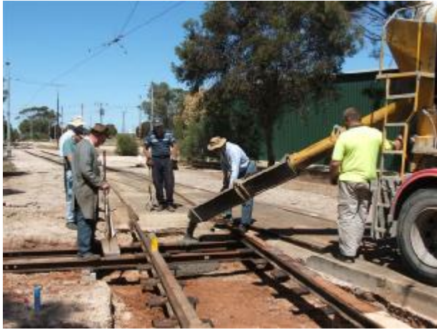
On hand for the concrete pour on Friday 9 Nov. 07 were Michael Bosworth, Bruce Lock, Mark Jordan, Michael Crabb, Ian Seymour and John Pennack. Chris Summers
