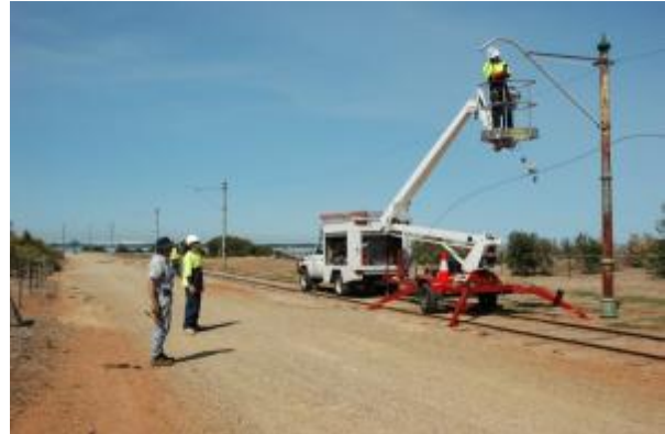
The work crew cuts the last span wire to bring down the overhead on the unconcreted section of track to the old terminus at St Kilda. Mike Bosworth watches on from the side. Friday 19 February 2010.
