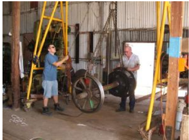
The wheel set is then removed from the trolley and lowered. The channel railway is then removed and doors shut.
