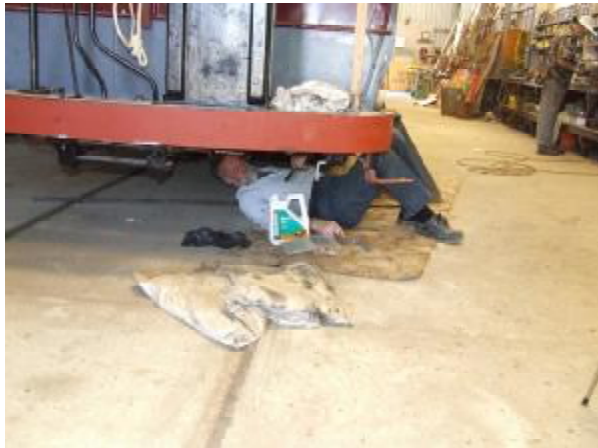
Jack Pennack installing retaining brackets under No. 14 to support and hold the electrical cabling.
