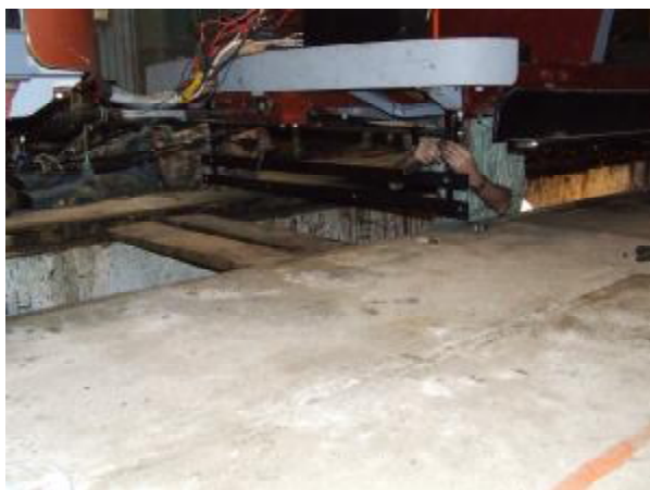
Bruce Lock and Charlie Rodgers installing the completed inner end lifeguard gate on No. 15.
