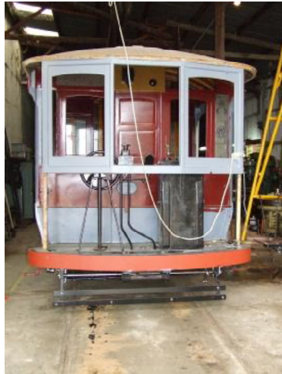
The eastern end of No. 14 showing the newly installed lifeguard and gate.
