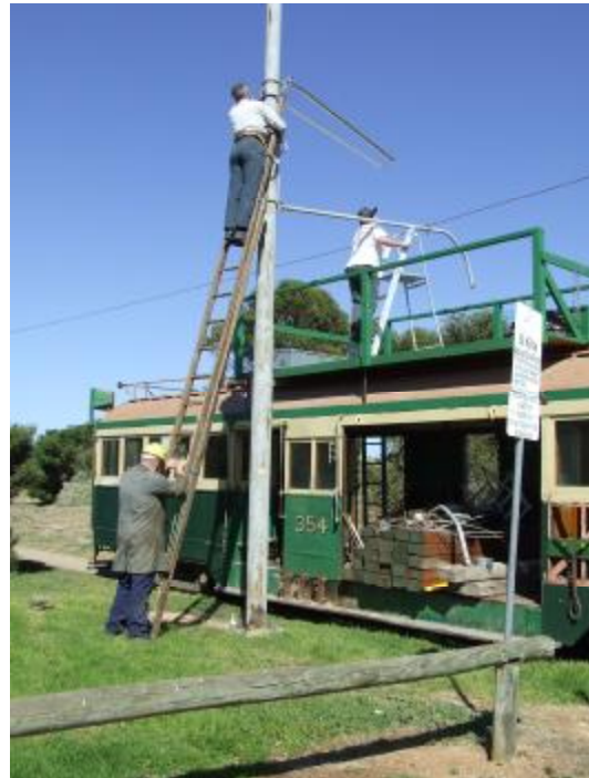
Ian Seymour, Jack Pennack and William Adams installing a bracket arm on the replacement Pole 43 in Shell Street.
