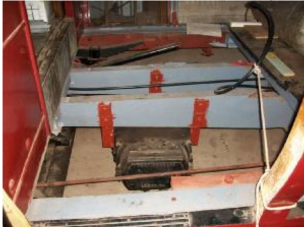
The Westinghouse DH10 compressor mounted under the drop end of A Type No. 15. Ian Seymour
