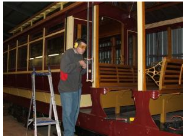
New AETM member Andrew Gilbertson (transferring from Sydney Tramway Museum), installing hand rails in the open (toast rack) area of 118. on Friday 5 June 2009.
