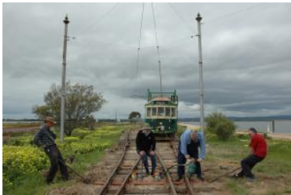
Mark Jordan, Jack Pennack, Kym Smith and Charlie Rodgers hard at work replacing point timbers at Mangrove Loop on Saturday, 11 Sep 10. Andrew Gilbertson
