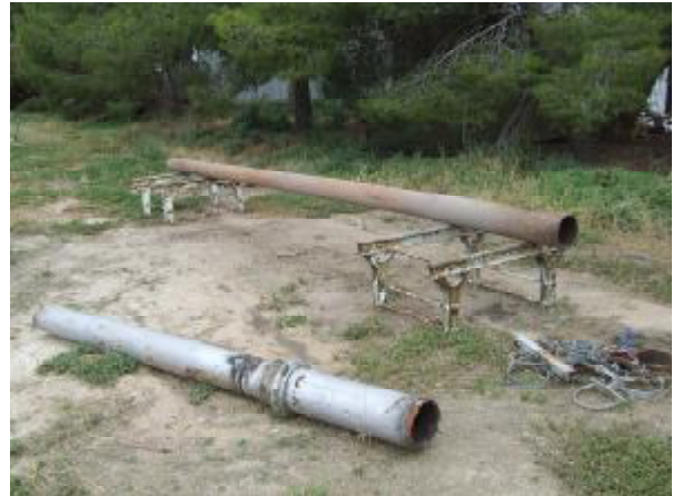
A pole that has been wire-wheeled to remove the old paint awaits priming. This pole is intended to be the replacement pole for Pole 8. Part of the original Pole 8 is in the foreground, and will be cut to provide the insert to weld inside the replacement pole to allow it to be welded to the stump of the old pole.
