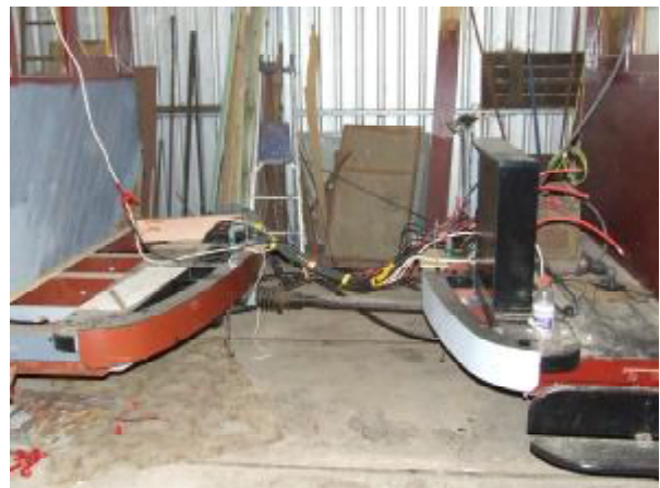
The spring-compensating towbar installed between 14 and 15. Keen-eyed observers will also note that most of the temporary resistor banks that were on the cab floor of tram 15 are no longer there, as they are now permanently installed under the trams.
