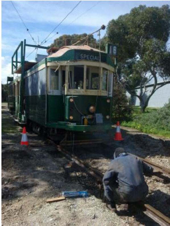
Bruce Lock welding a rail joint on the section being prepped for concreting on Friday, 10 Sep 10. Andrew Gilbertson
