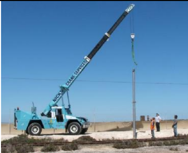
Andy Hall and Michael Bosworth watching a replacement pole being put in place on the lakeside track.
