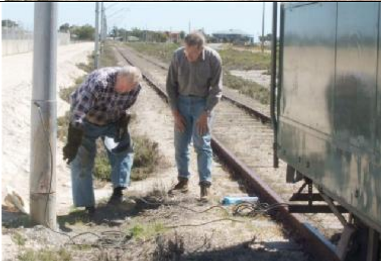
Bruce Lock preparing to weld the pole into position watched by Michael Bosworth.
