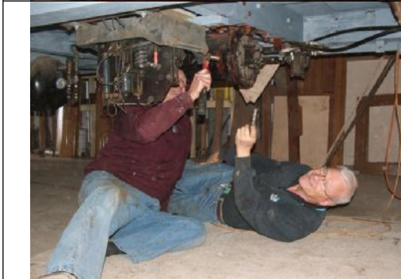
Bruce Lock and Michael Crabb installing brake equipment under car 118. Chris Summers 03 AETM Aug
